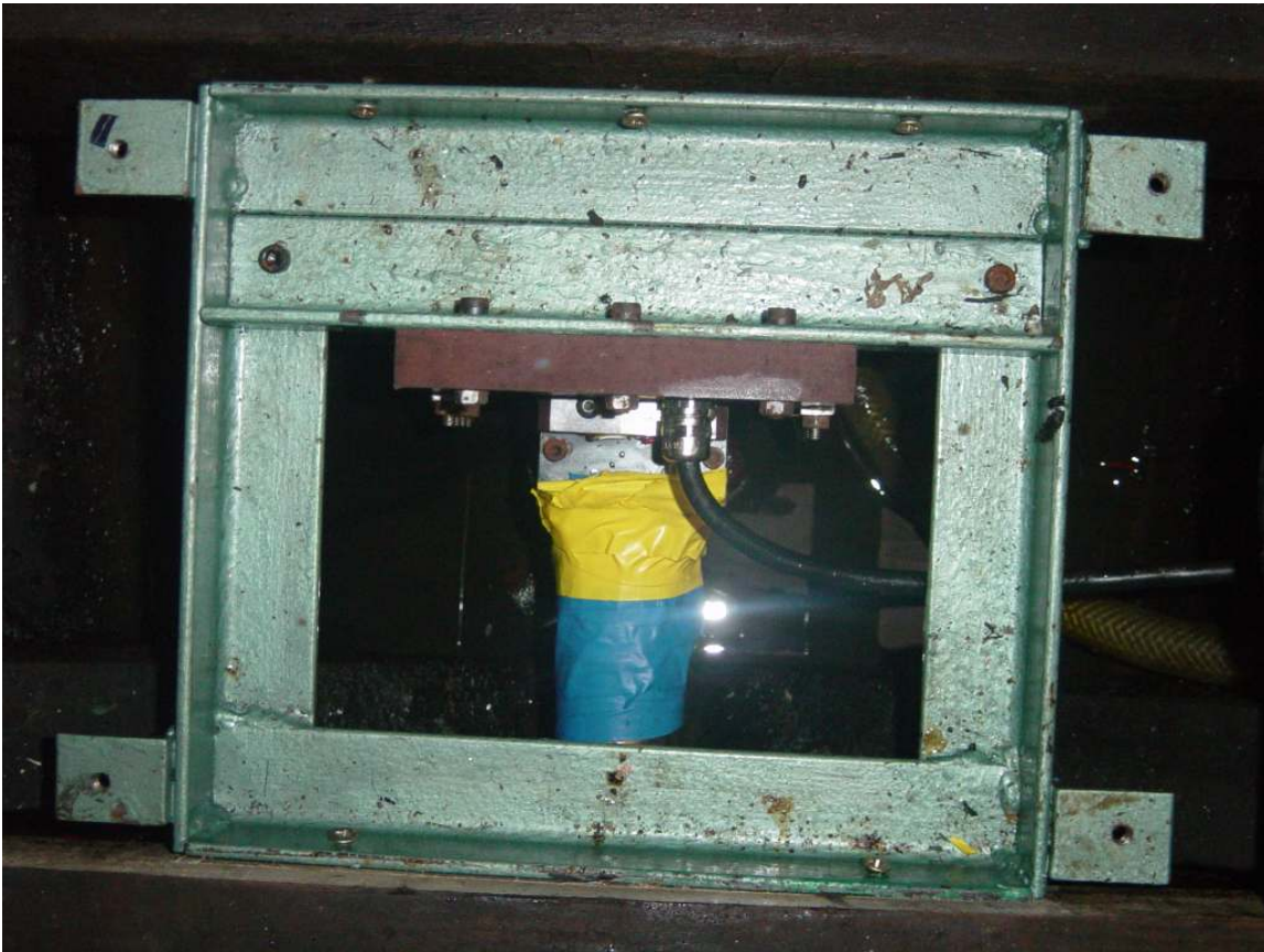
Figure 04: Ma Gandole torque sensor after initial installation on 14 th December 2006.
