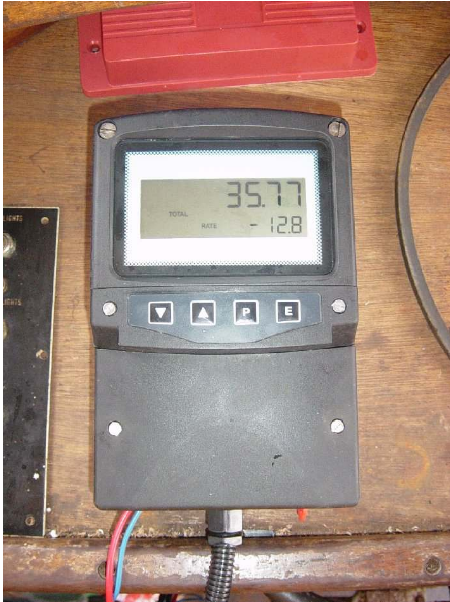
Figure 03: Instantaneous fuel flow meter installed on Ma Gandole bridge
