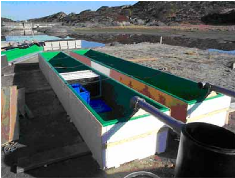
Image 4 The insulated treatment troughs, with “drop-in” modules
