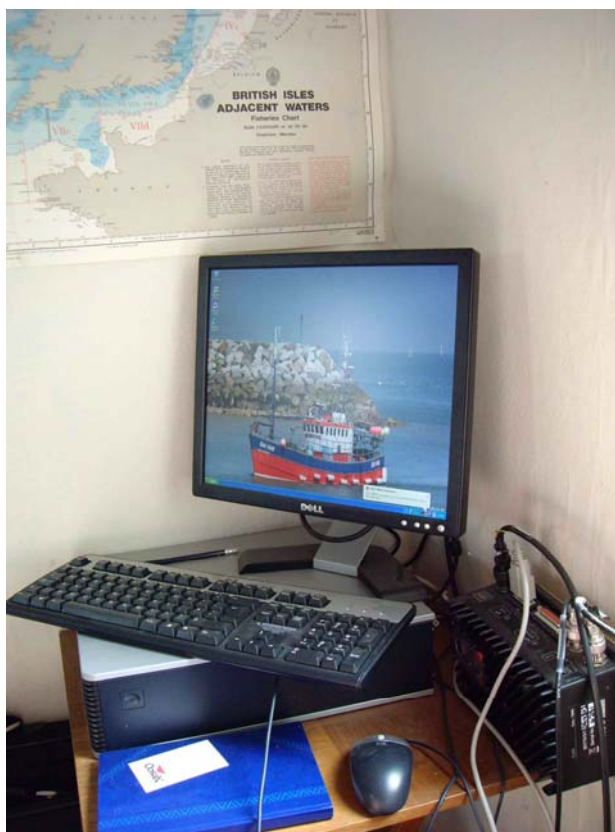
TDMA Base Station at Newlyn Office
