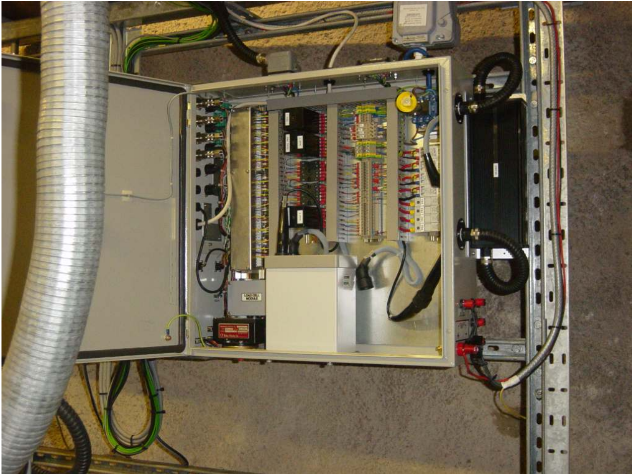
Figure 4: Data logging and control hardware
