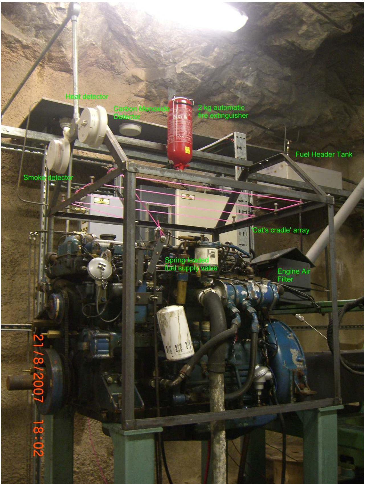
Figure 8: Test engine showing fire protection measures installed to support unattended operations for prolonged testing.
