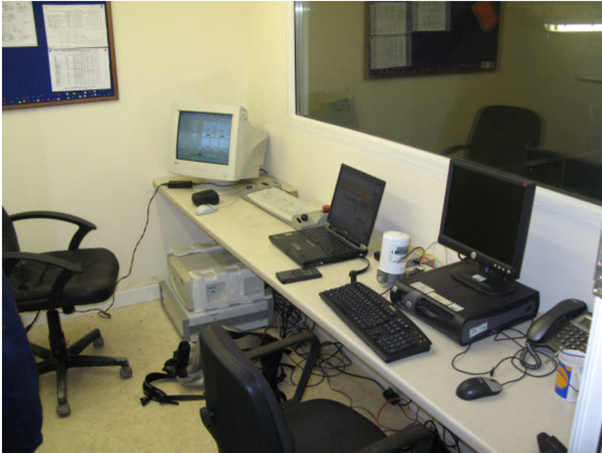
Figure 11: Control room showing CP Engineering instrument rack on floor beneath computer screen
