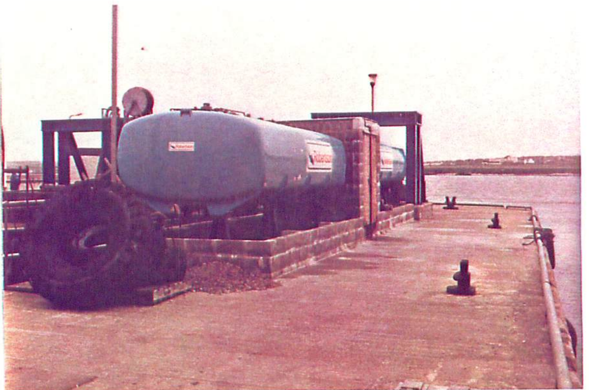
Photo 4 : New fuel tanks alongside the Ro-Ro berth.
