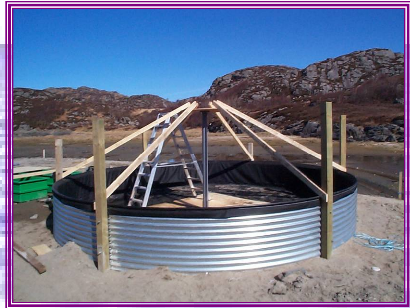
A 5m diameter circular tank being installed, with its own light-proof cover
