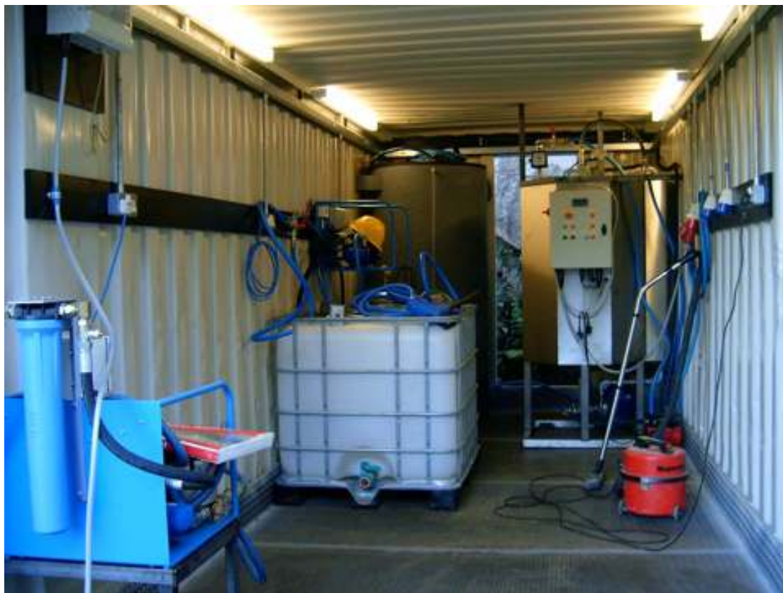
Figure 4: Containerised biodiesel batch reactor plant, close to commissioning stage.
