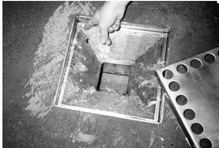
Figure 35 - Separator Catch Basket in the Drain with the Cover Removed
