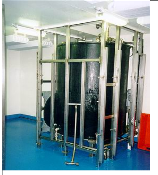
Figure 3 - Pumpable ice tank in fish room of a white fish trawler
