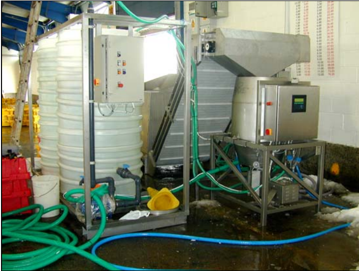
Figure 25 - Trials of ground/crushed ice system on market (brine maker to left, ice maker at front on right , with ice silo behind
